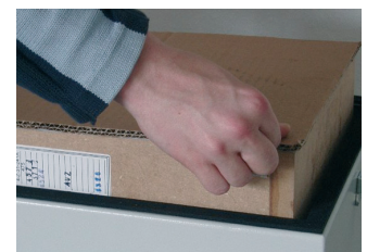
contamination free replacement of the filters
